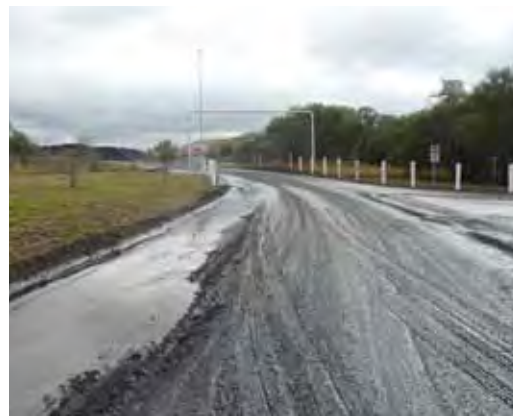
^ Coal-sediment contaminated mud along Pikes Gully Road, Liddell
